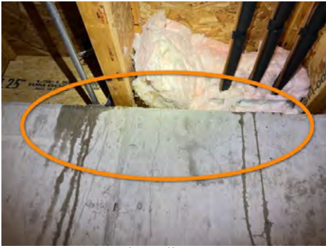
Basement North wall
