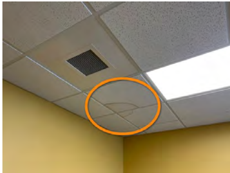
Northwest office- previous leaking
