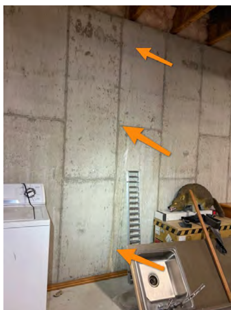
Basement North Wall
