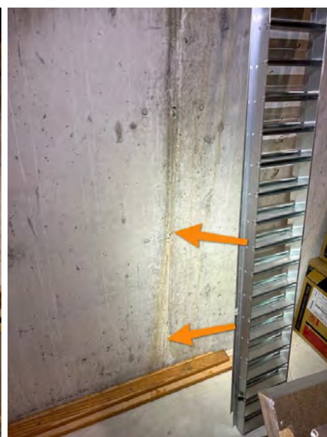
Basement North Wall
