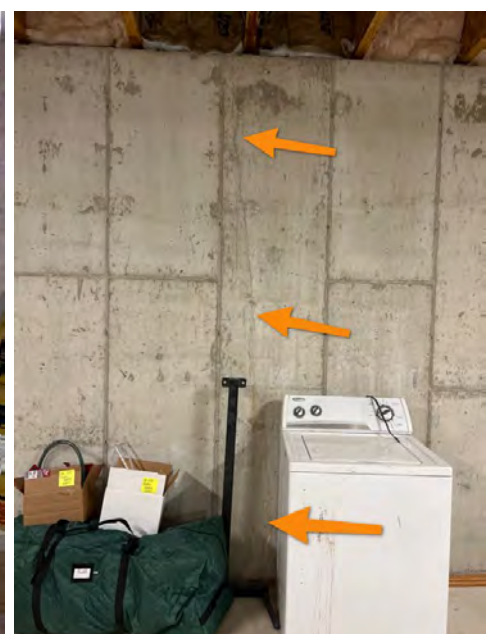
Basement north wall
