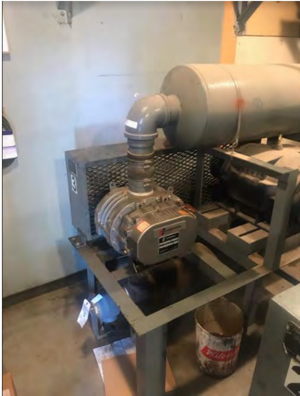
#3 blower before removal
